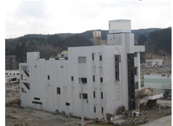
Tsunami evacuation building that withstood tsunami - 200m from the coast - Flood water depth was more than 13m.
