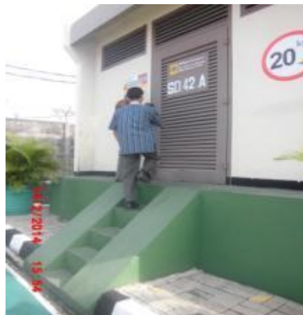
Figure 9. Substation building that has been raised (ASTRA Daihatsu Jl. Danau Sunter Utara)
