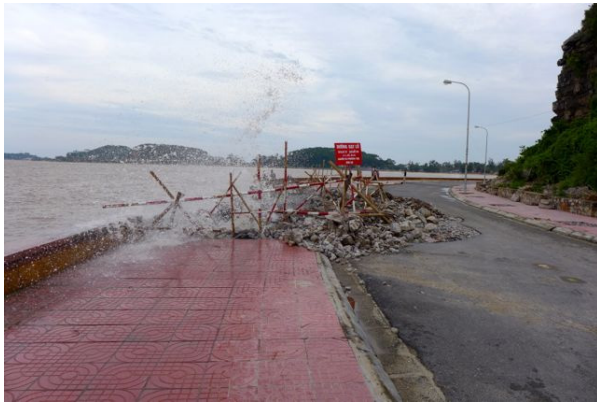
Photo 6.6 Coastal dyke damaged at Do Son Area (Unknown if the damage caused by Typhoon No. 5 JEBI:JEBI(2013))
