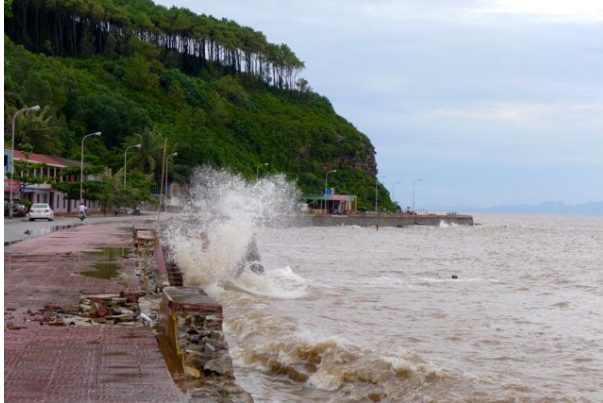
Photo 6.4 Coastal dyke damaged at Do Son Area (Unknown if the damage caused by Typhoon No. 5 JEBI:JEBI(2013))
